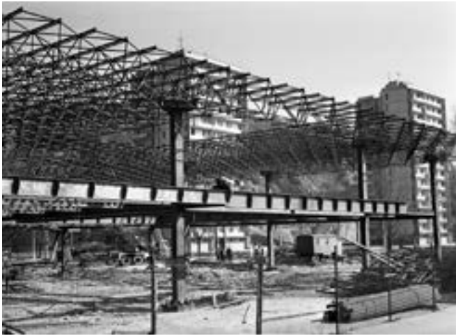
CONSTRUCTION OF THE BUILDING OF THE OFFICE OF THE CHIEF ARCHITECT OF BRATISLAVA, 1968
